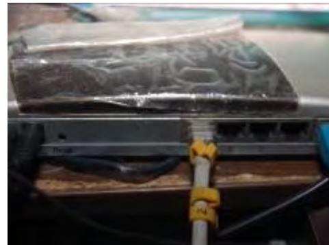
(b). Network Switch
