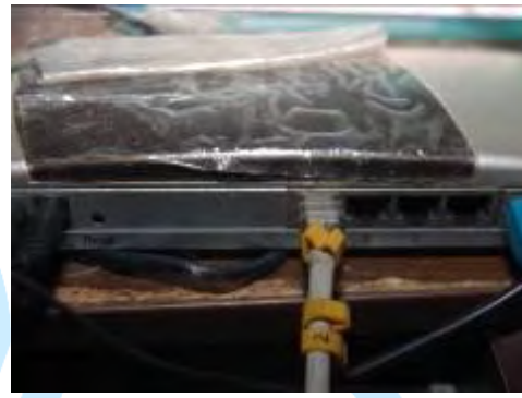
(b) Network Switch
