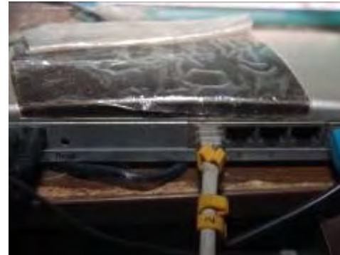
(b). Network Switch
