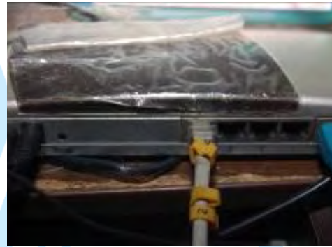
(b). Network Switch
