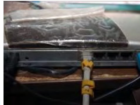
(b). Network Switch
