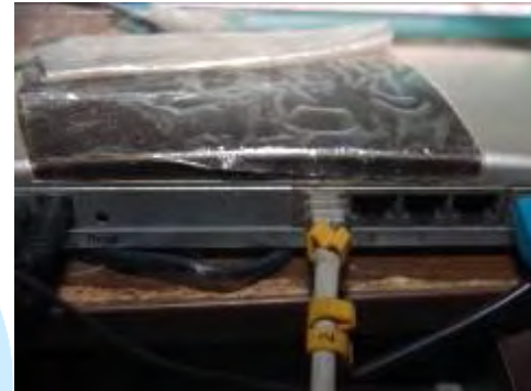
(b). Network Switch
