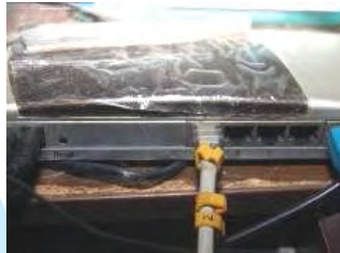
(b). Network Switch
