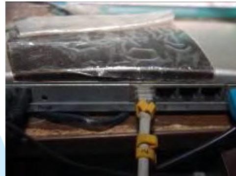
(b). Network Switch
