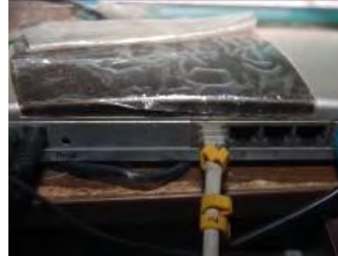
(b). Network Switch
